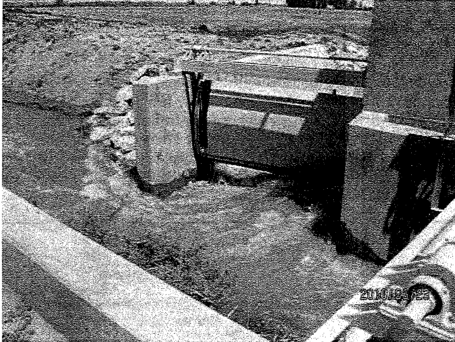
South Side ADS new bifurcation control structure. Back when there was river flow, Water can be seen flowing under the return gate headed back to the river.
