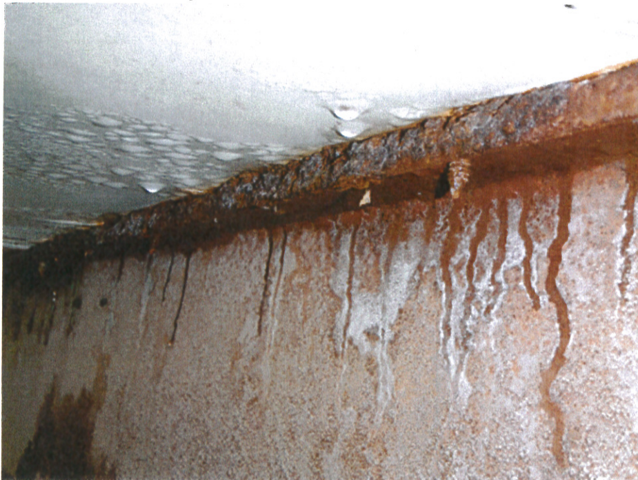
Detail view of corroded roof purlin
